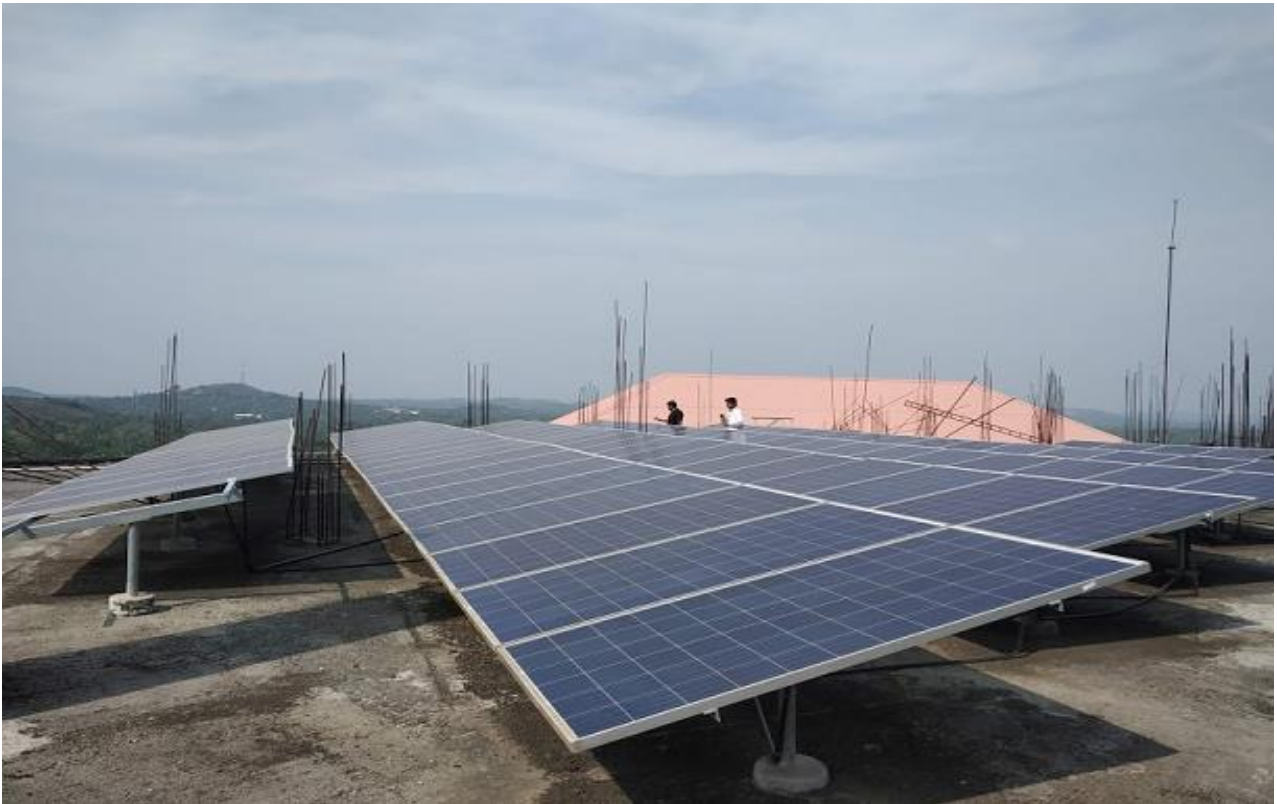
30KW SOLAR POWER PLANT
